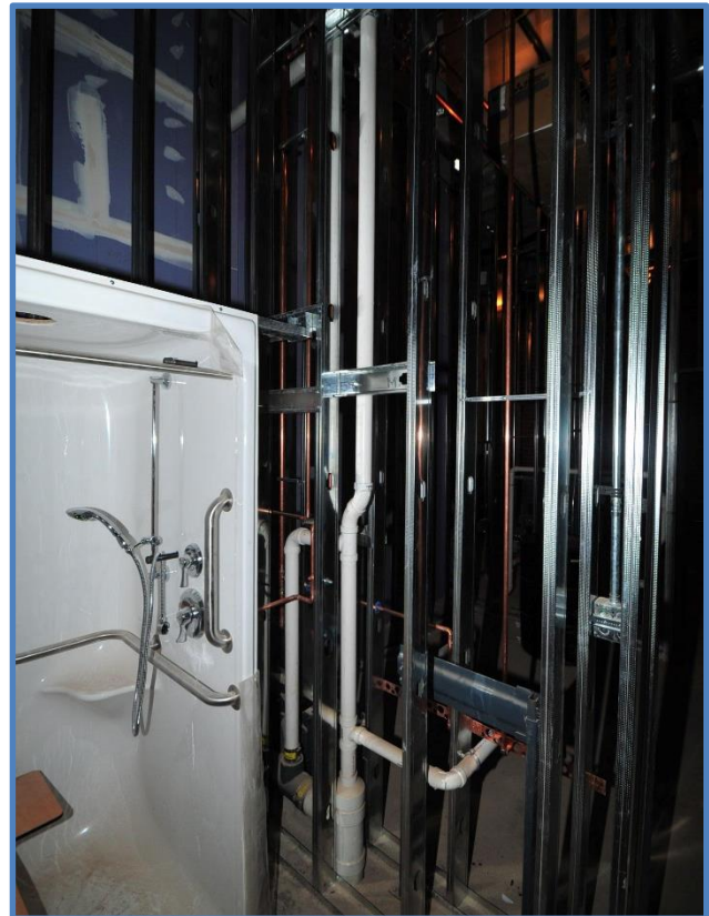
Figure 3: Example of MEP milestone photo. (Multivista®)
