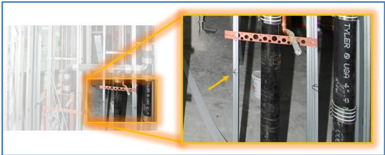
Figure 9: Photographic evidence of missing handrail blocking. (Multivista®)
